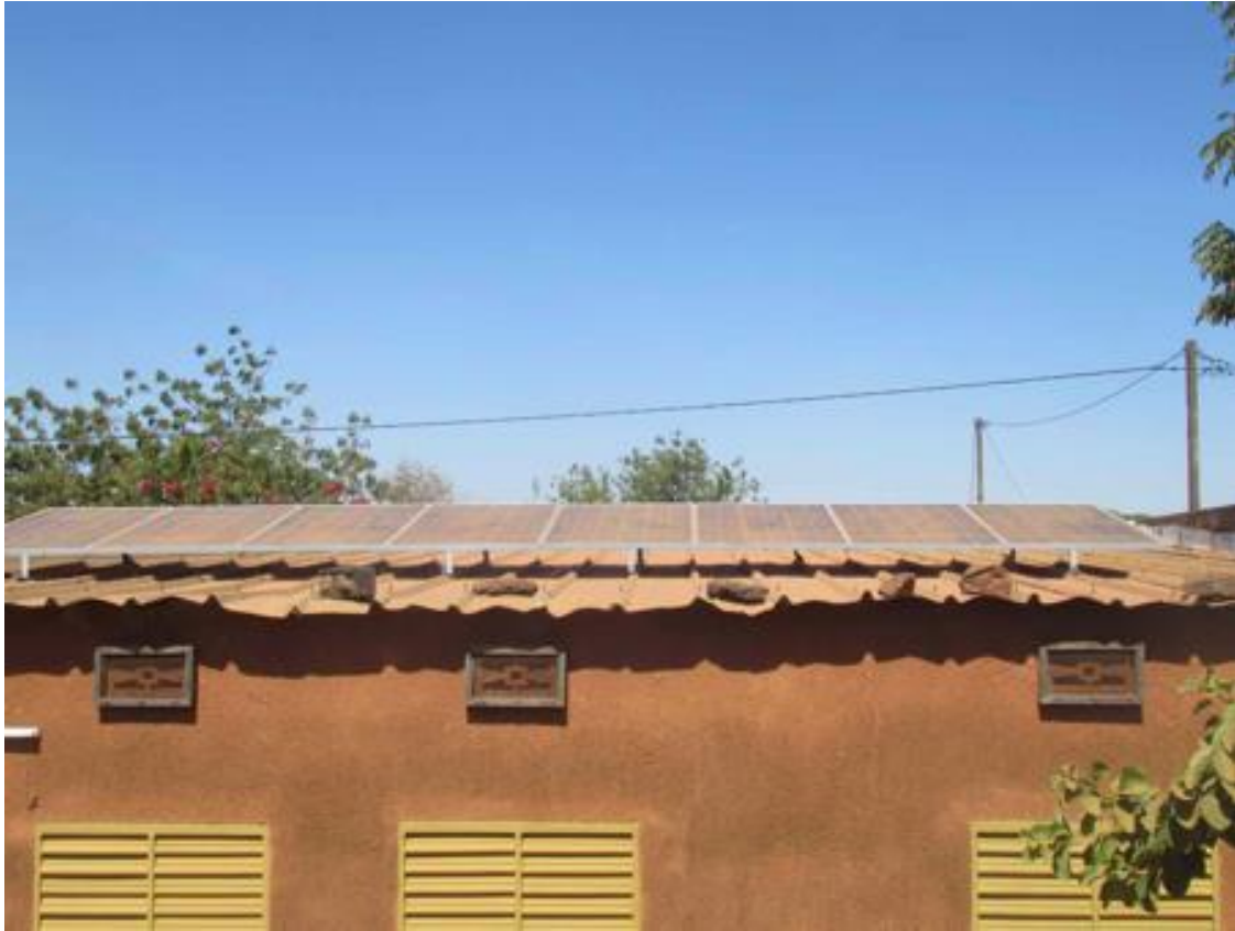
Eight solar panels on the roof
